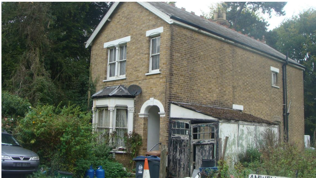
Picture 13. The Folly Amwell Lane. An early 20th century property whose site appearance could be much improved. Selected features such as the bay window and its detailing are worthy of retention and possible additional protection.
