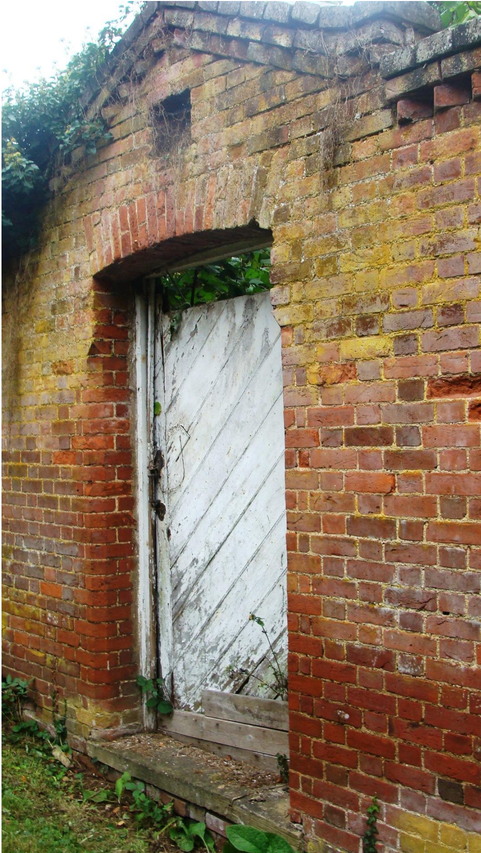
Picture 26. Wall and door adjacent to footpath 16 would benefit from repairs.
