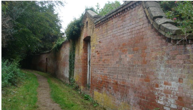
Picture 15. A fine brick wall important and visually prominent in the public domain adjacent to a well used footpath. As can be seen some repairs necessary and consideration should be given to the removal of selected vegetation.
